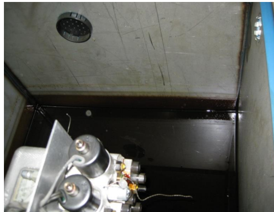
Sludge/varnish deposited on inside of tank and also found in the operating valve
